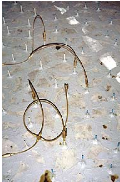
Fig. 22: Injecting one port at a time would make for a very long day. A manifold installed at the end of a line allows several ports on the same crack to be injected simultaneously
