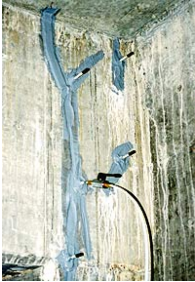
Fig. 15: Leaks in a crack seal are quickly located by injecting air into the crack
