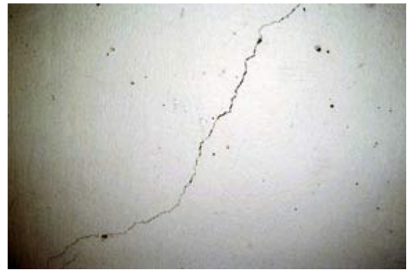
Fig. 5: Packing the existing crack is not a good option for this thin crack
