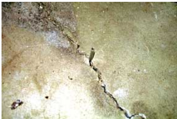
Fig. 13: Cracks that are at least 1/8-in. (3-mm) wide are candidates for insertion porting
